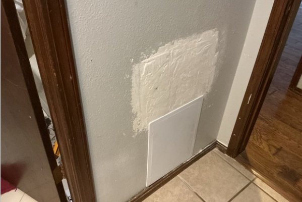
804 Drywall for recent plumbing access hall needs to be repaired
